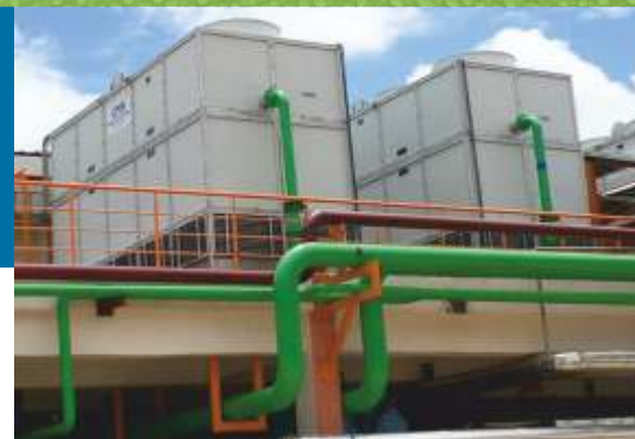
Installation at United Breweries Unit - Chamundi (1250 kW X 3 Nos.)
