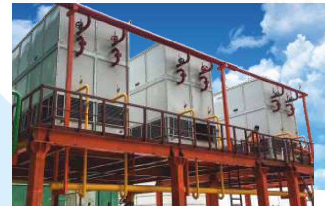
Evaporative Condenser Installation with De-Super Heating Coil at Carlsberg, Mysore
