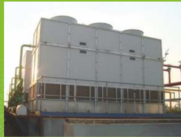
Installation at Venkateshwara Hatcheries at Davangere (900 kW X 4 Nos.)
